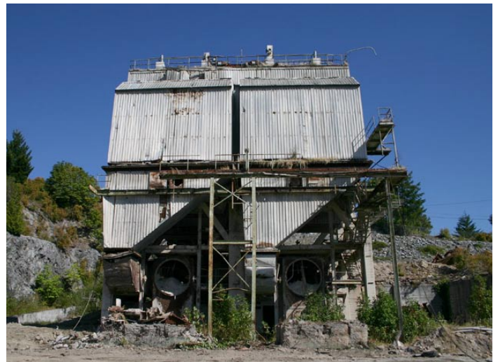
Once key to the production of concrete, these derelict precipitators were deconstructed in preparation for the environmental remediation process.
